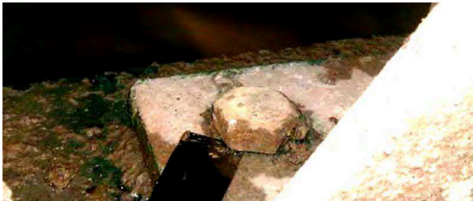
Fig. 5 - In this mill there were lock washers which had corroded away. Any fasteners that have failed should be replaced with stainless steel lubricated if they were mild steel standard fasteners.
