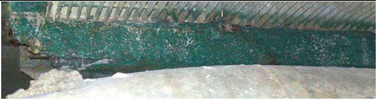
Fig. 6 - The end of this walkway support is entirely corroded through and much of the material is completely gone. There is also delamination in process on other parts of the support. This part will need to be replaced.
